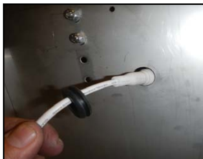
Picture 33.0: Cable and Grommet
