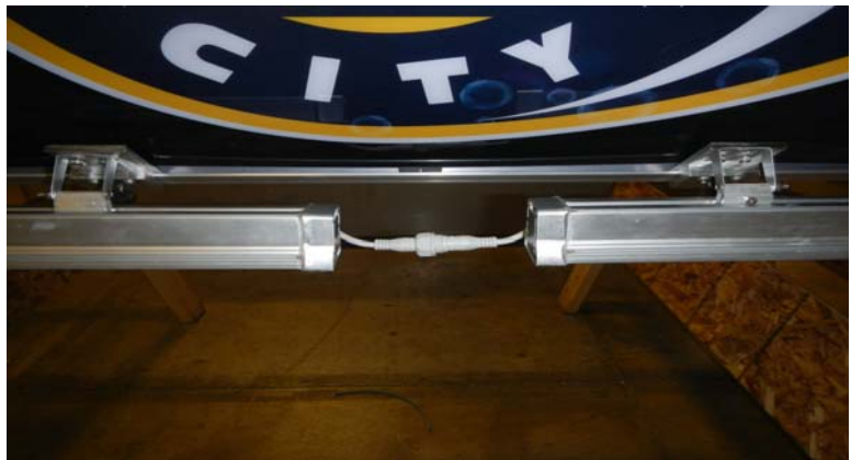
Picture 31: Light Bars Connected Together
