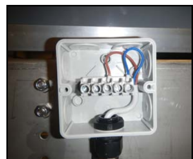
Picture 34.0: Junction Box Installed
